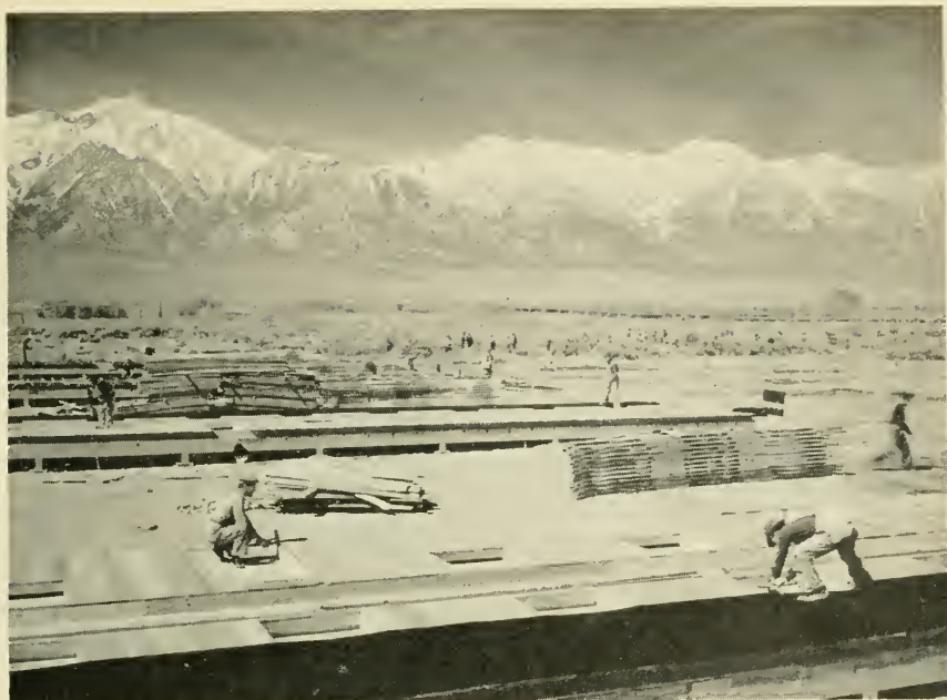
Carpenters are at work building quarters for evacuees at Manzanar, Calif., with the high Sierras in the background.
