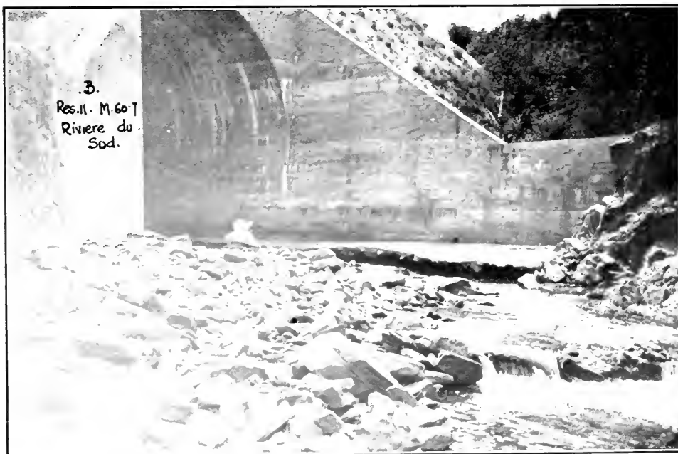
District B, Residency 11. Mileage 60.7. 40 Foot Concrete Arch over Riviere du Sud. Page 120.
