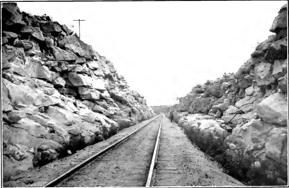
District F, Residency 31. Rock Cutting at Mileage 39.0. Note width of excavation where men are Standing. Page 70.
