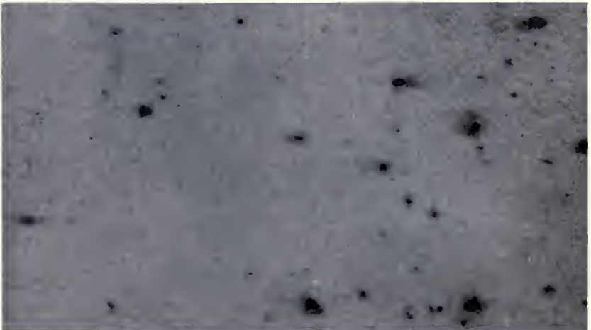
Photographic reference standard Number 8 — type 1, rusting not accompanied by blistering. This standard has often been recommended as the "repaint stage." Photo courtesy American Society for Testing Materials. (See literature citation 12.) (Fig. 4)
