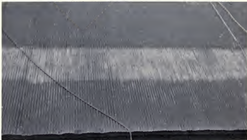
The top portions of the bottom sheets of Panels 46 through 81 on the north side were wire brushed before painting. These panels were 100 percent rusty (see Fig. 2). (Fig. 10)
