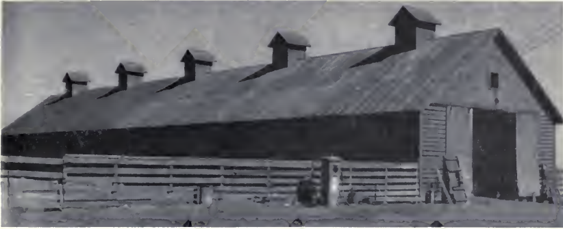
North side of crib before painting. The one-third of the roof at the left (Panels 46 through 81) was 100 percent rusty. (Fig. 2)
